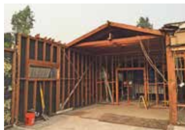
Most interior walls are taken down to the studs, for all new wiring.
